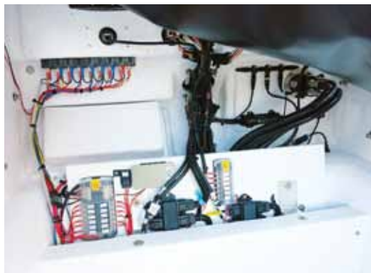
Very few leisure boats can boast wiring of this clarity and competence.
