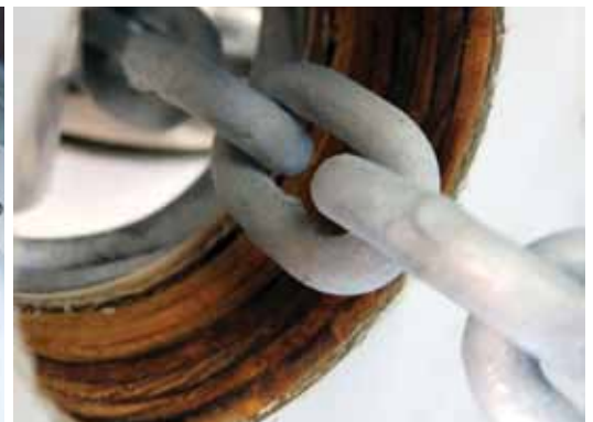
The unprotected plywood edge below the windlass needs protecting.
